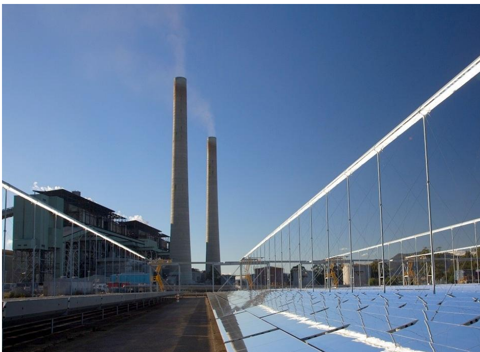
Figure 2 Novatec's solar boiler at Liddell, coal-fired power station, Australia
