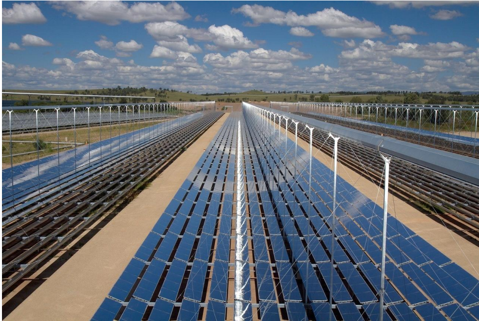
Figure 1 Novatec's solar boiler at Liddell, coal-fired power station, Australia
